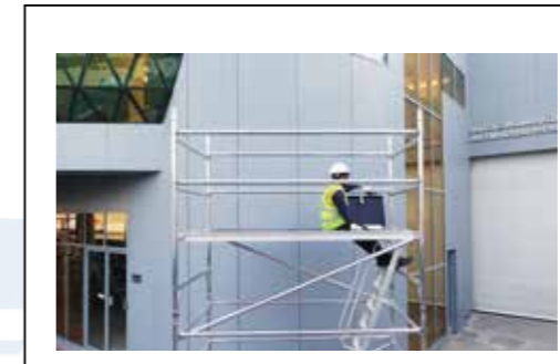
STEP-9 Sitting on the trapdoor opening of the platform fit two horizontal brace on both the open sides of the platform.
