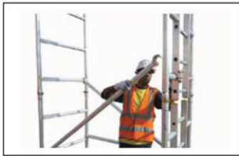
Step 6 Position diagonal braces YELLOW colour coded From the first rung of both frame in a zig zag pattern from 1 st to 3 rd rung & 3 rd to 5 th rung either side of the tower opposing each other as illustrated Make sure diagonal brace is aligned.
